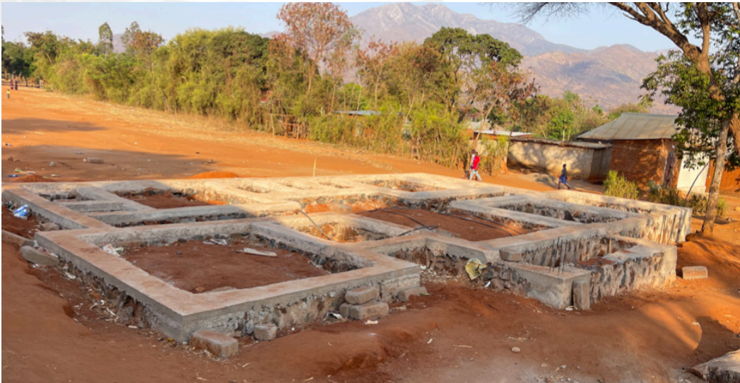
Picture 4: A police station reportedly under construction by citizens in Chamkorama Ward, Kongwa District Source: Field data, 2023
