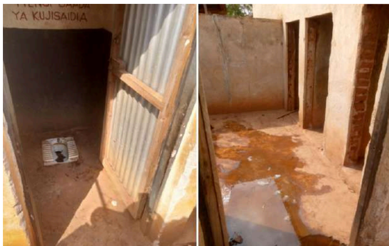
Picture 4: Condition of toilets at Kambarage and Jitegemee Primary Schools in Morogoro
