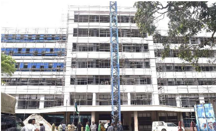
Picture 30: Ongoing construction of a new hospital building of the Mjini Magharibi Regional Hospital – August 2022
